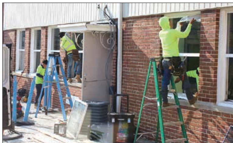
St. Mary's School installed new windows for its classrooms this summer, getting the building ready to welcome back students!
